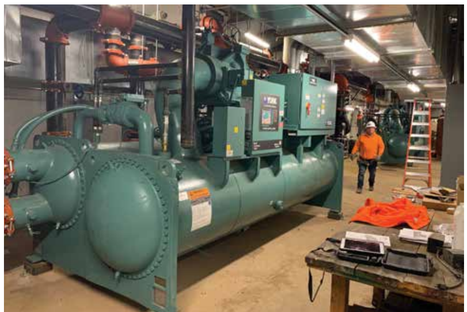
Working in existing facilities can be challenging, and the installation of this chiller was no exception, requiring well-planned rigging and the removal of two walls.
